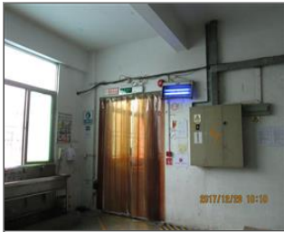
Photo of fire safety equipment Emergency exit sign and emergency light and fire alarm.JPG
