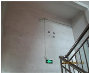
Photo of fire safety equipment Emergency light and evacuation indication sign.JPG
