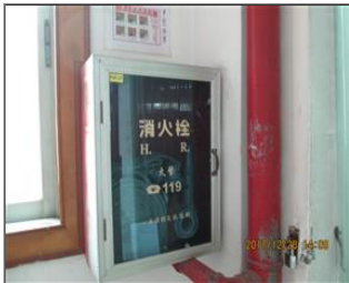
Photo of fire safety equipment Fire hydrant.JPG
