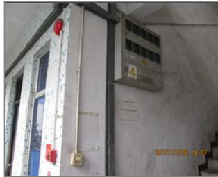
Photo of the dormitories (if applicable) Fire alarm.JPG
