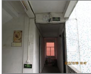
Photo of the dormitories (if applicable) Evacuation indication sign and exit sign.JPG
