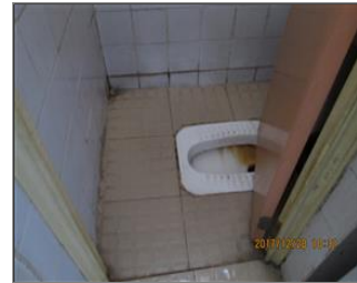
Photo of the sanitary facilities Washing room.JPG
