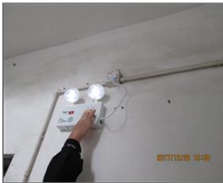
Photo of fire safety equipment Emergency light testing.JPG
