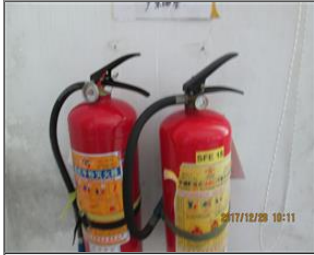
Photo of fire safety equipment Fire extinguishers.JPG
